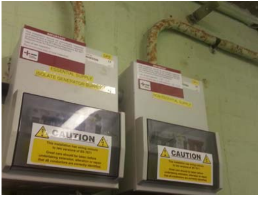
The newly certificated fuse boards.
