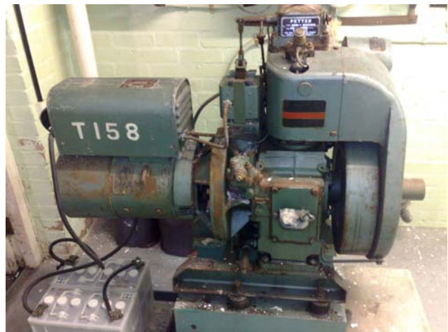
The 3kW Standby Generator.
