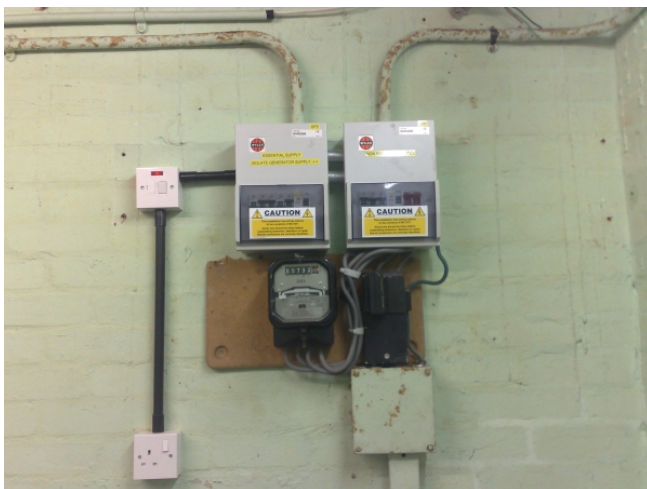
The new modern distribution boards kindly donated by Wilts Electrical
