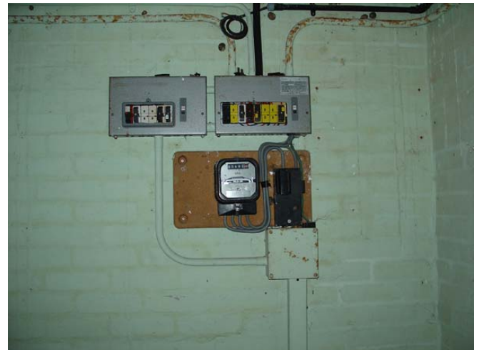
The Original Electrical distribution board.
