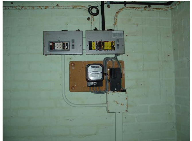
The Original Electrical distribution board.
