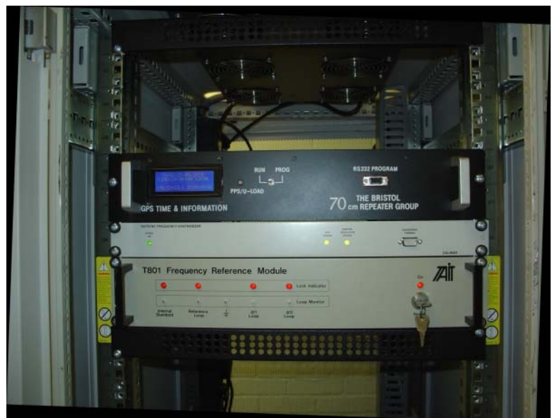
New GPS Clock unit at the top, GPS frequency standards below
