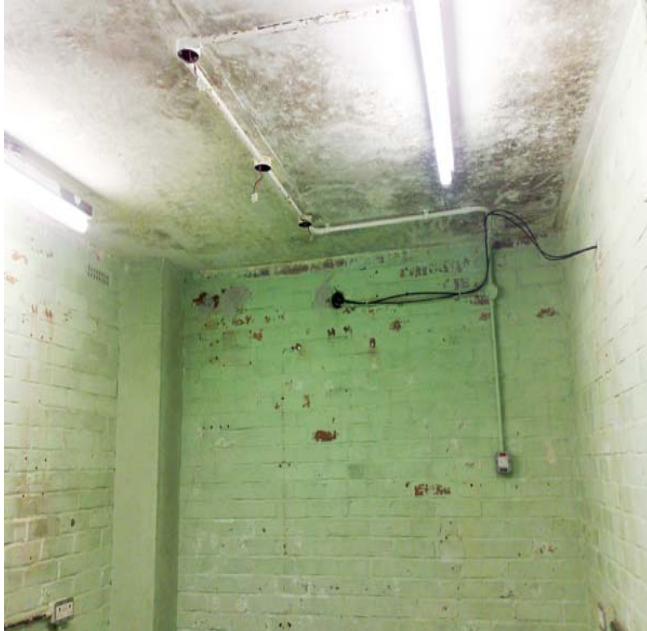
Comms room just after we took ownership
